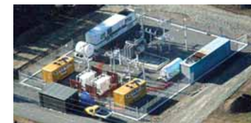
Temporary generation provided by Marlborough Lines while Transpower installed the new conductors for the third 110kV Stoke to Blenheim circuit.
